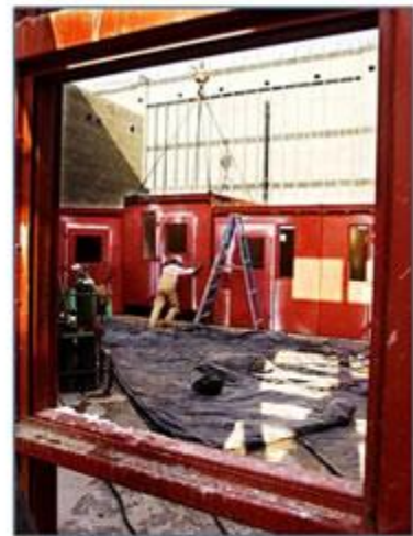
An idea that cells James Frazier of Sweeper Metal Fabricators Corp. helps guide a prefabricated jail cell into place at the new Creek County Jail. Each cell weighs 6,000 pounds and is painted and ready to occupy once plumbing and electrical systems are attached. STEPHEN HOLMAN / Tulsa World
